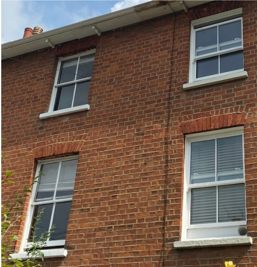
The replacement uPVC sash windows at no. 33 (right) next to the timber sash windows at no. 31 (left) which is the adjoined building in the terrace
