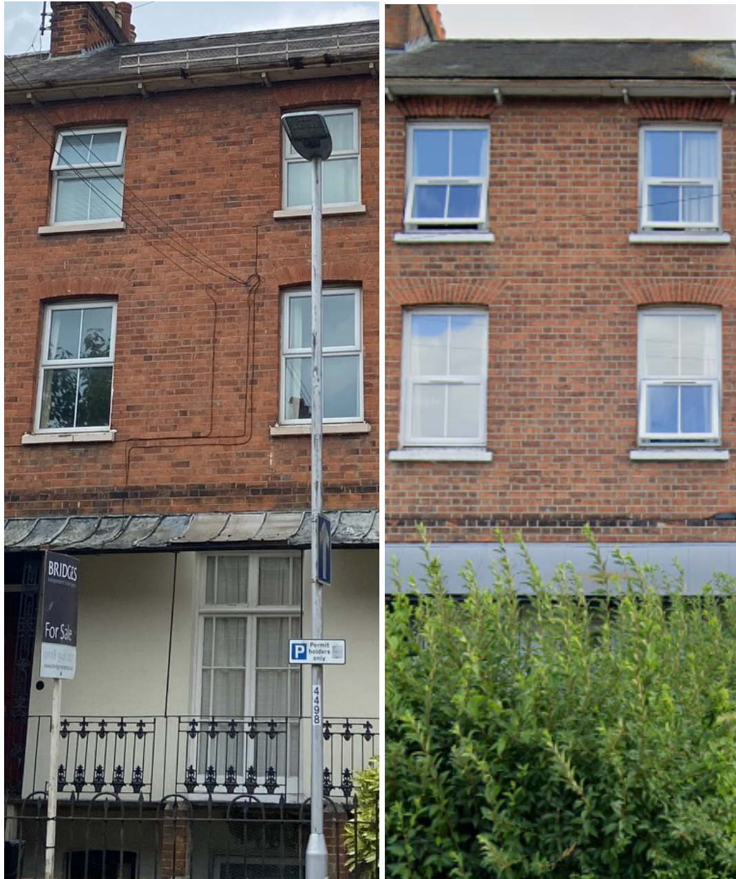
Poor quality replacement non-sash style uPVC windows elsewhere within Jesse Terrace
